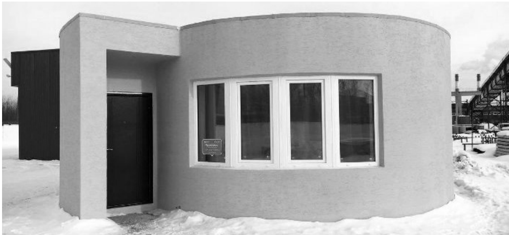
Fig. 4: Russian Company Apis Cor Built this House in just 24 Hours using their Concrete 3D Printer
